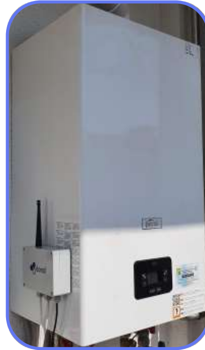
Boiler attached with the heating controller
